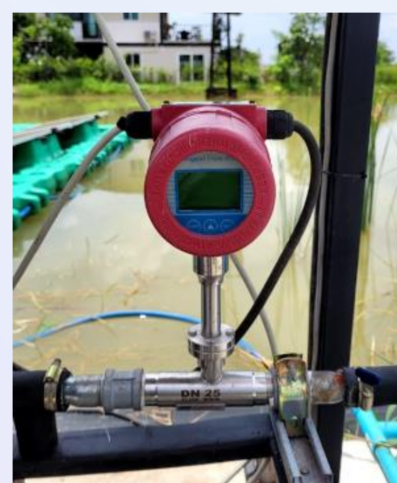
Air flow meter
