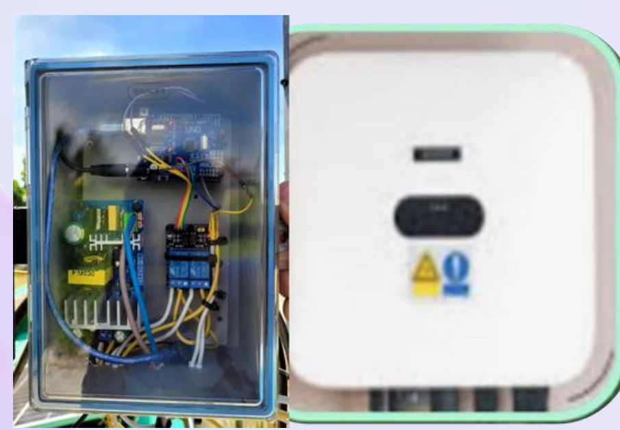
(2) DC/AC inverter and controller units
