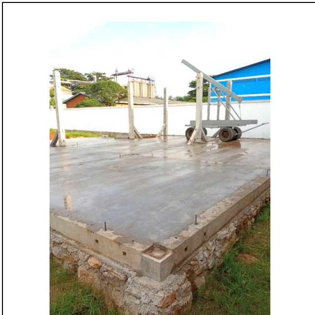
Hand crane raising posts on the ground slab. Foldable mini tower cranes may be considered for a quicker construction
